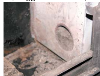
(Plugged Clean Out)
