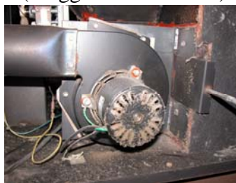
(Plugged Exhaust Fan)
