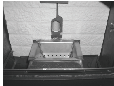
Wood Pellet Firepot Installed
